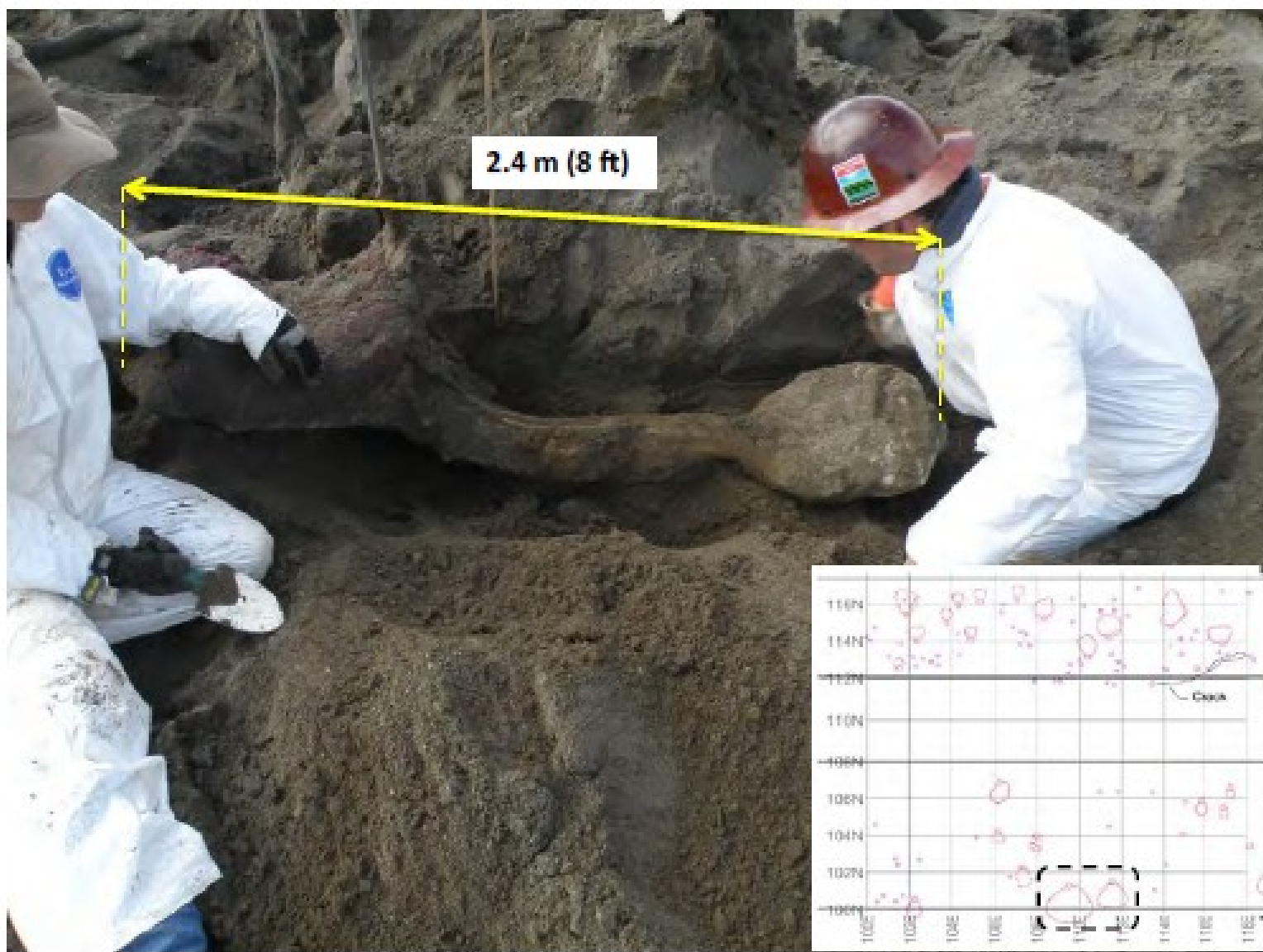
Figure 5-2. Continuation of waterside burrow into the levee on the sandy levee
