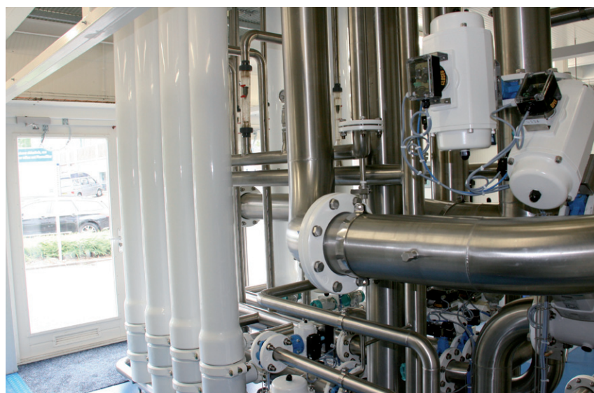
FIGURE 2.5 MBR SKID WITH THE MEMBRANES SET UP OUTSIDE OF THE BIOLOGICAL TANK
