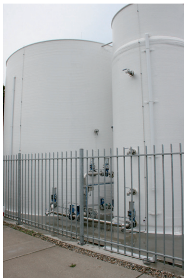
HYDROLYSIS TANK AND DIGESTER
