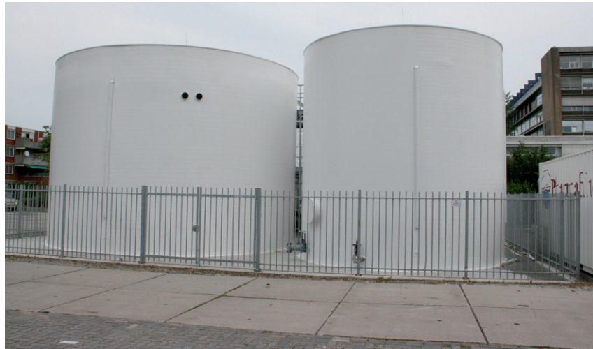
FIGURE 2.4 MBR TANK (L) AND DIGESTER (R)
